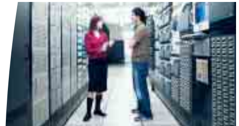
Data centres: server rooms, communications centres, data storage units, network equipment.
